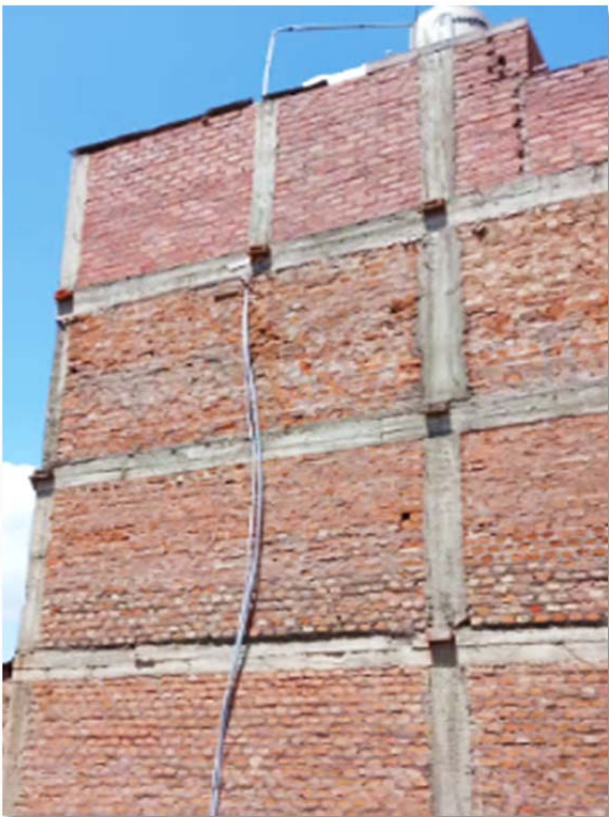
Figure 11. Absence of confinement elements
