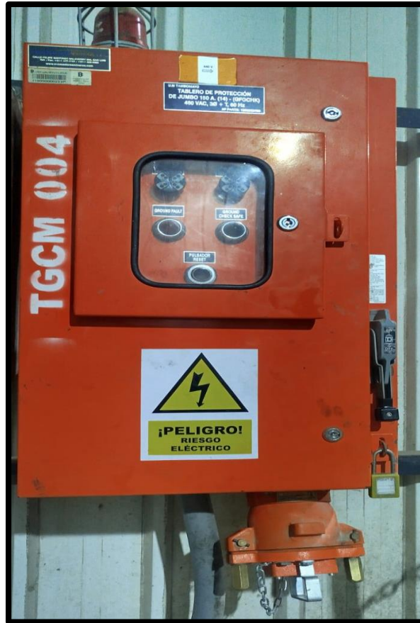
Figura 21. Tablero Ground Fault y Ground Check.
