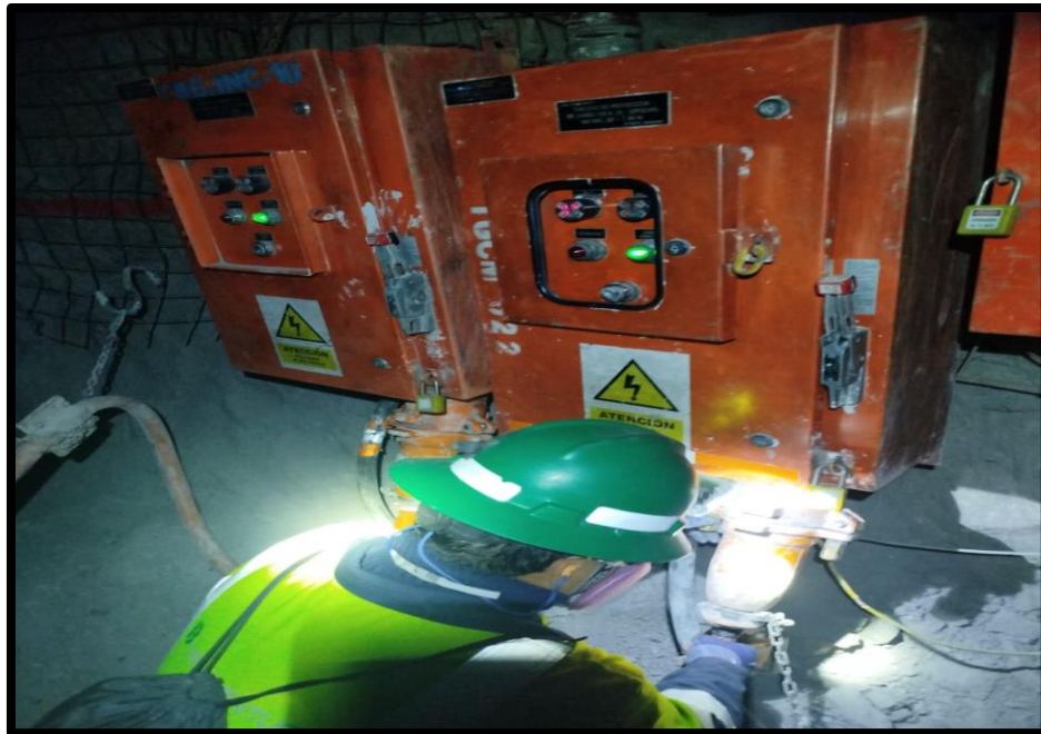
Figura 8. Tablero Ground Fault y Ground Check.
