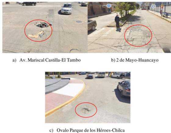
Figure 1. Deterioration of rigid pavement in Huancayo
